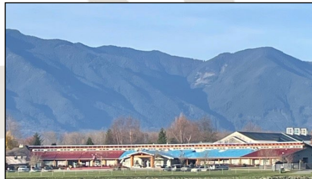
Metal roof in the process of being installed at the Stó:lō Elders Lodge.
